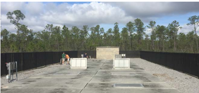
30,000 GPD decentralized treatment system
