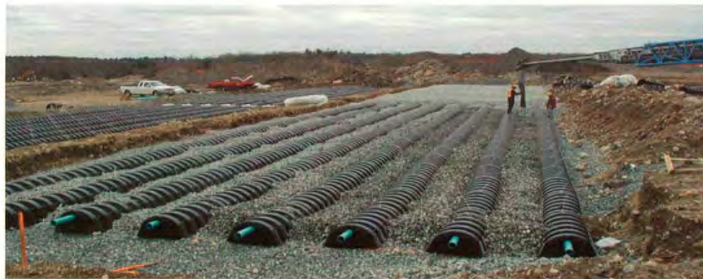
Infiltrator chambers are placed under a parking lot for an outlet mall. Highly treated wastewater is distributed within the chamber bed via a pressure distribution piping network.
