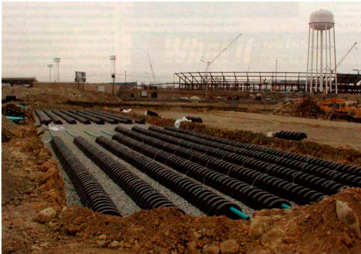
Infiltrator wastewater disposal chambers are installed under parking lots at Gillette Stadium. Excess water is discharged below the surface of the parking lots by a series of chamber beds, allowing recharge of the local aquifer.
