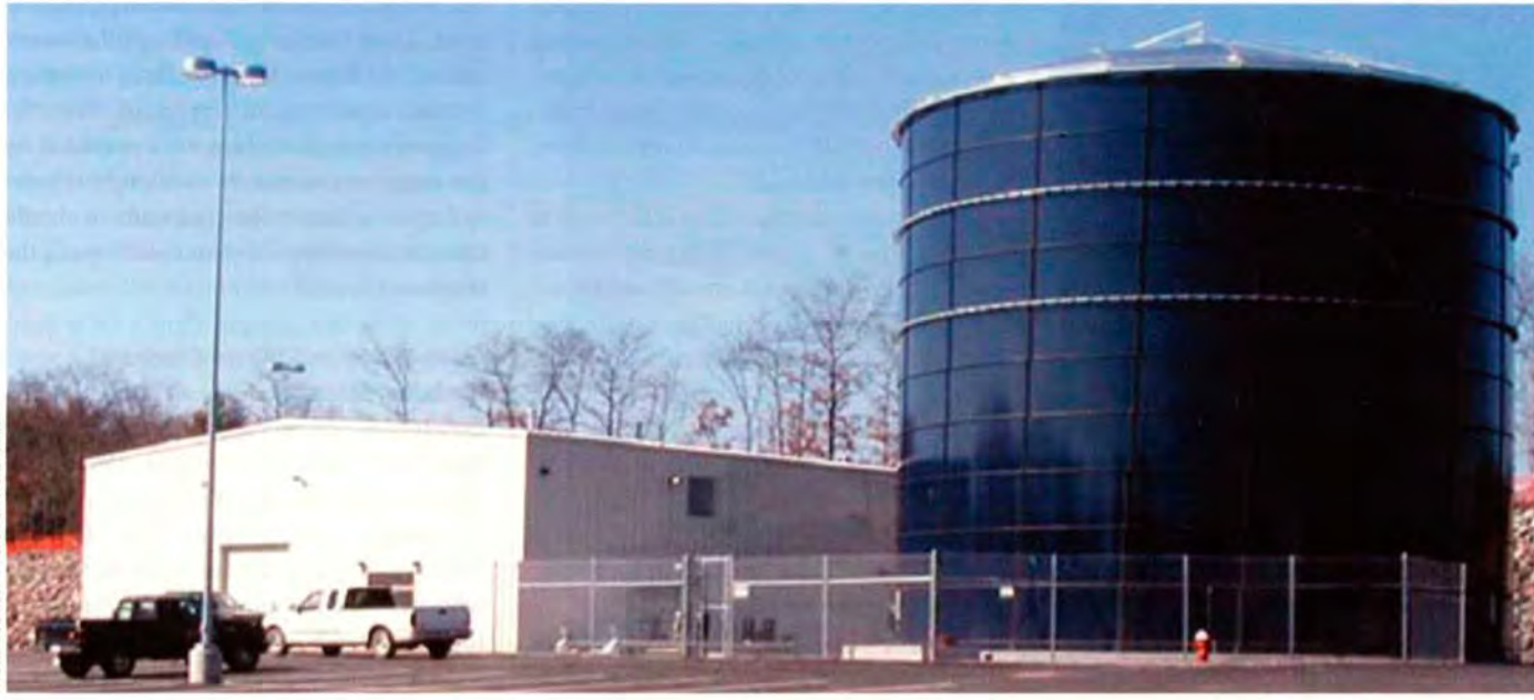
Gillette Stadium water reclamation facility and flow equalization tank
